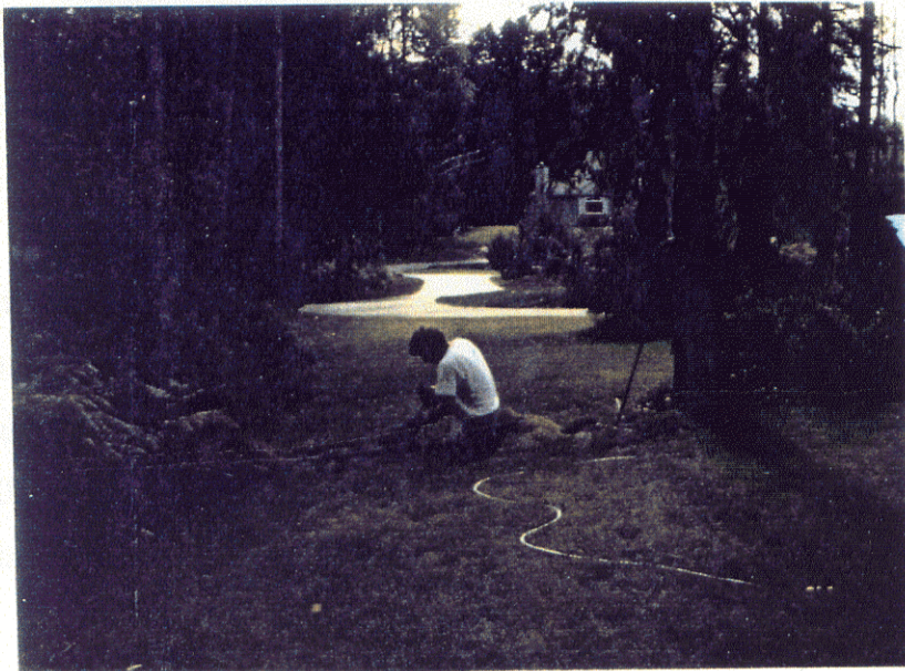
Figure 3.5: Union Hill infiltration trench during construction (above) and installation of piezometer (below)
